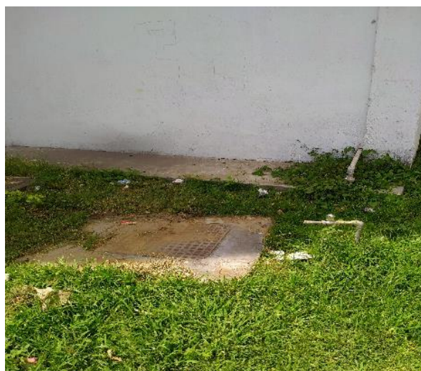
Rainwater Harvesting Tank
