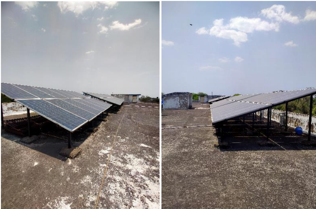
Solar Power System
