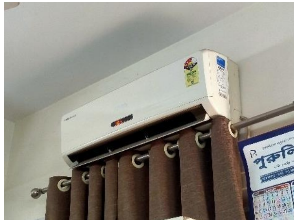
Air Conditioners used in the campus
