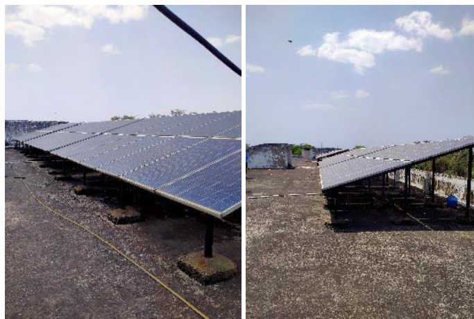
Solar Power Plant
