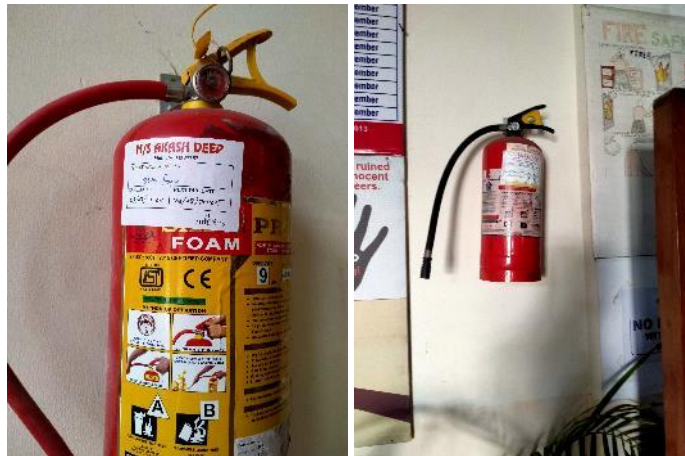
Fire extinguishers provided
